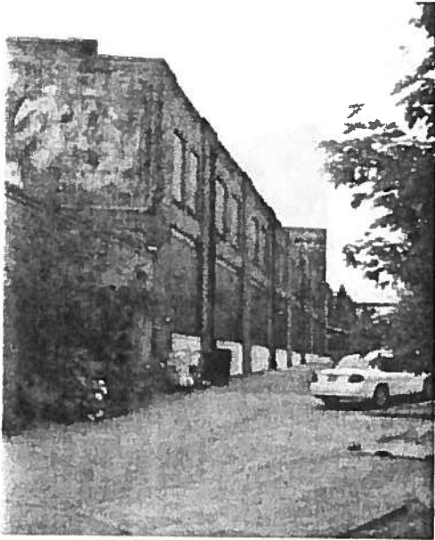
AUGUST 2007 view of the West (rear) facade. The rear bays once used for loading and unloading goods from the train are now completely boarded up in the vacant building. Source: Artifacts Consulting, Inc.
