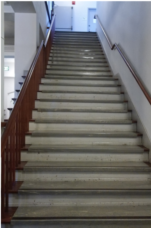
Figure 33. View looking up east stair of main stair hall. Note the covering on the treads and new handrails.
