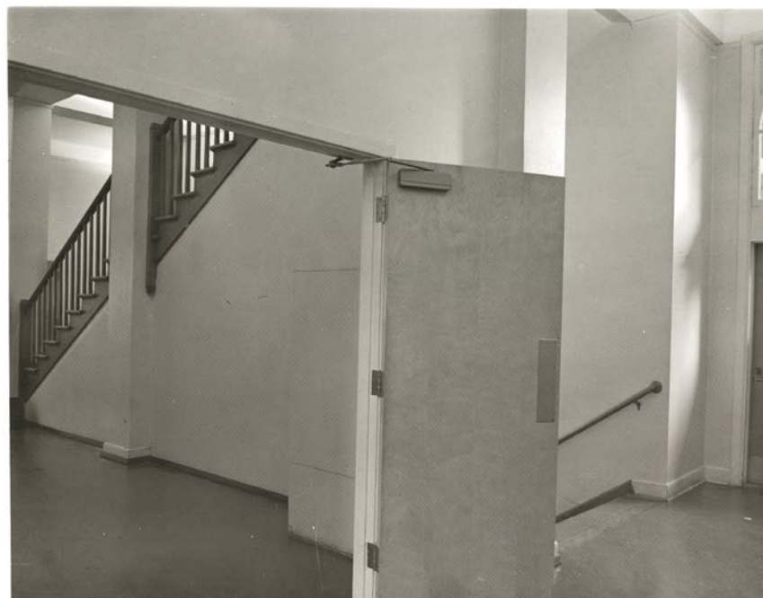
PARRINGTON HALL 2 ND. FLOOR CORRIDOR CONNECTING STAIRS AND FIRE EXIT 5-29-74 AI-1491 PHOTO NO 6
