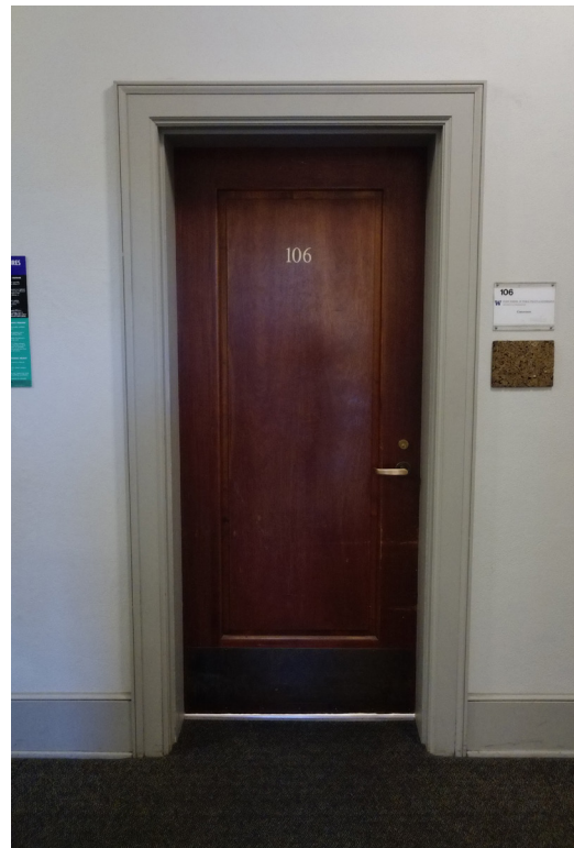
Figure 34. Example of replacement doors present throughout the building.
