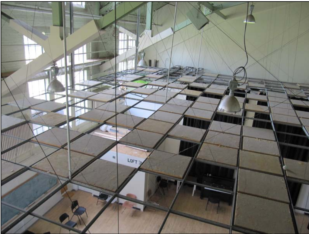
Views of two large spaces on the back (east side) of the former Main Gymnasium space, showing the tall windows, exposed mechanical and ceiling systems, and fire-resistant cladding on the roof trusses.
