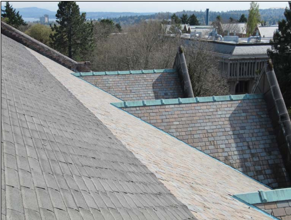
View of the gabled roof over the main mass from the tower. Note the combination of gray-colored composition shingles (over the former skylight area) and multi-colored slates, the multi-colored slates on the dormer roofs, copper cresting on the dormer ridges and copper flashing.
