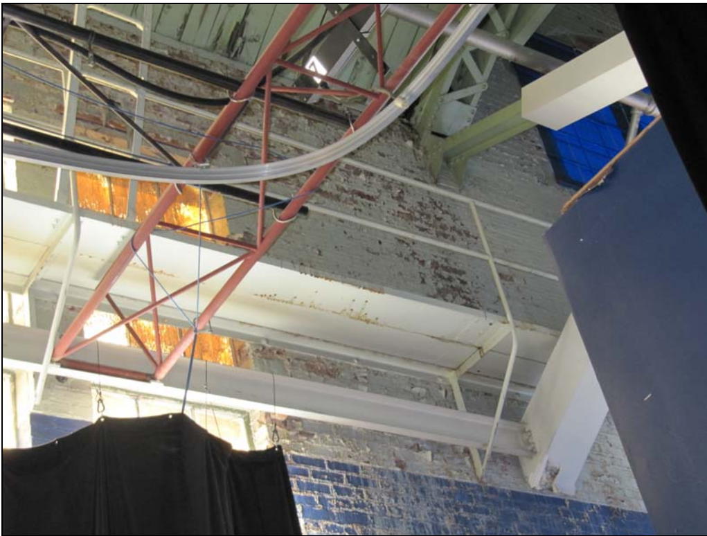
Top, finishes in the basement library space are relatively new. Directly above, a view of the perimeter masonry and spalled paint on the steel framing in Room 200, evidence of water infiltration from the roof and walls. Some of the wood roof decking appears to be damaged also.
