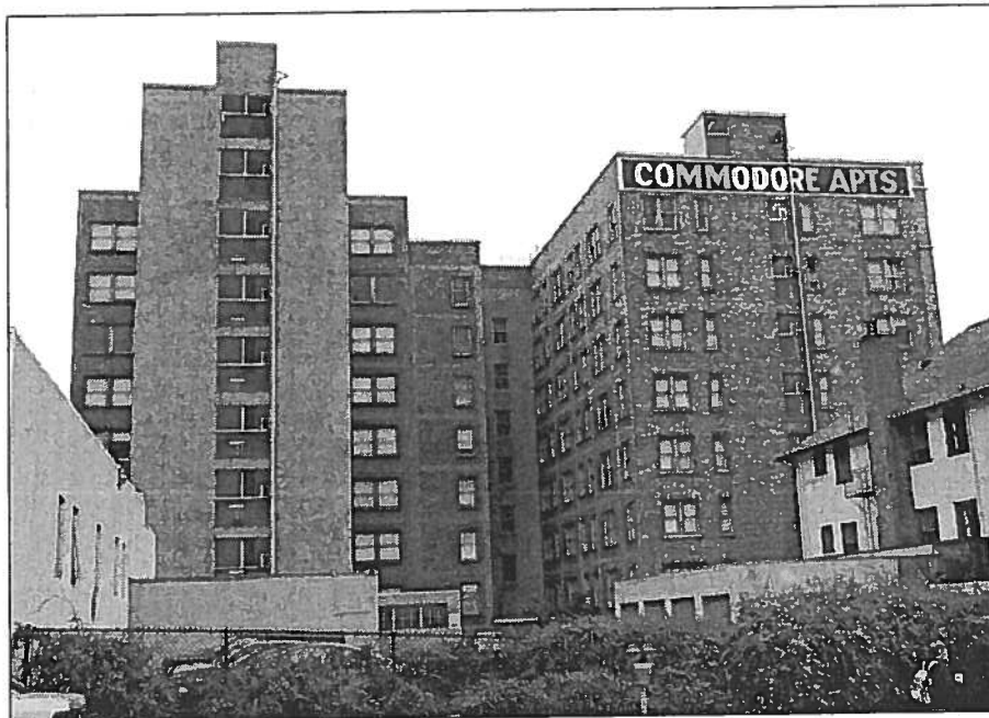
The Commodore Duchess Apartments, view of the west (back) facades, October 2004. Note the simple concrete exit stair mass, the exposed concrete frames, and the raised penthouse on these secondary facades.
