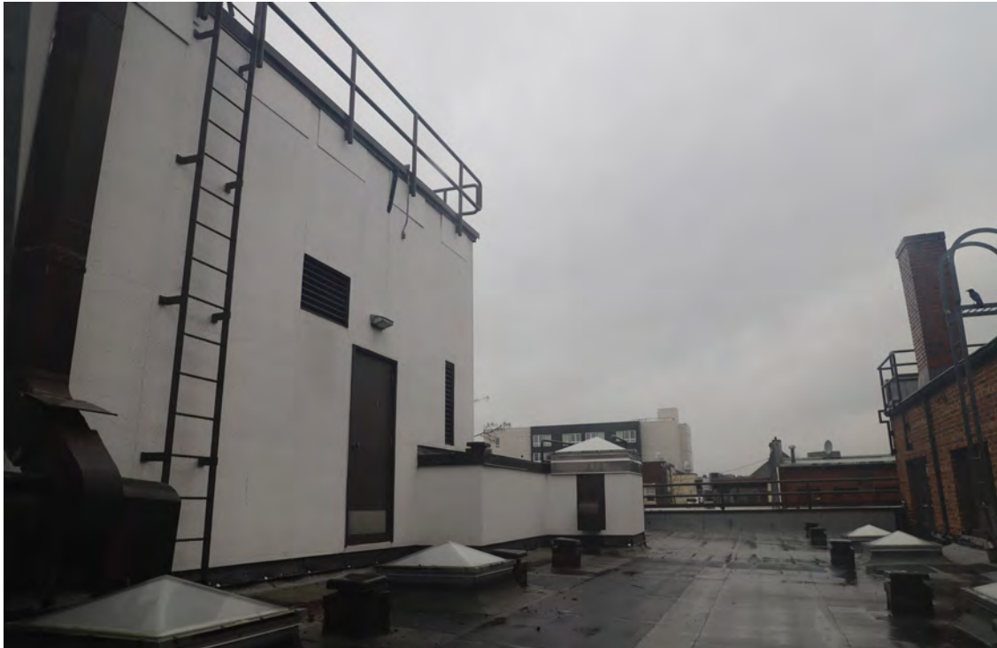
Figure 39. Roof over the southwest portion looking west. The south mechanical addition is visible at left.
