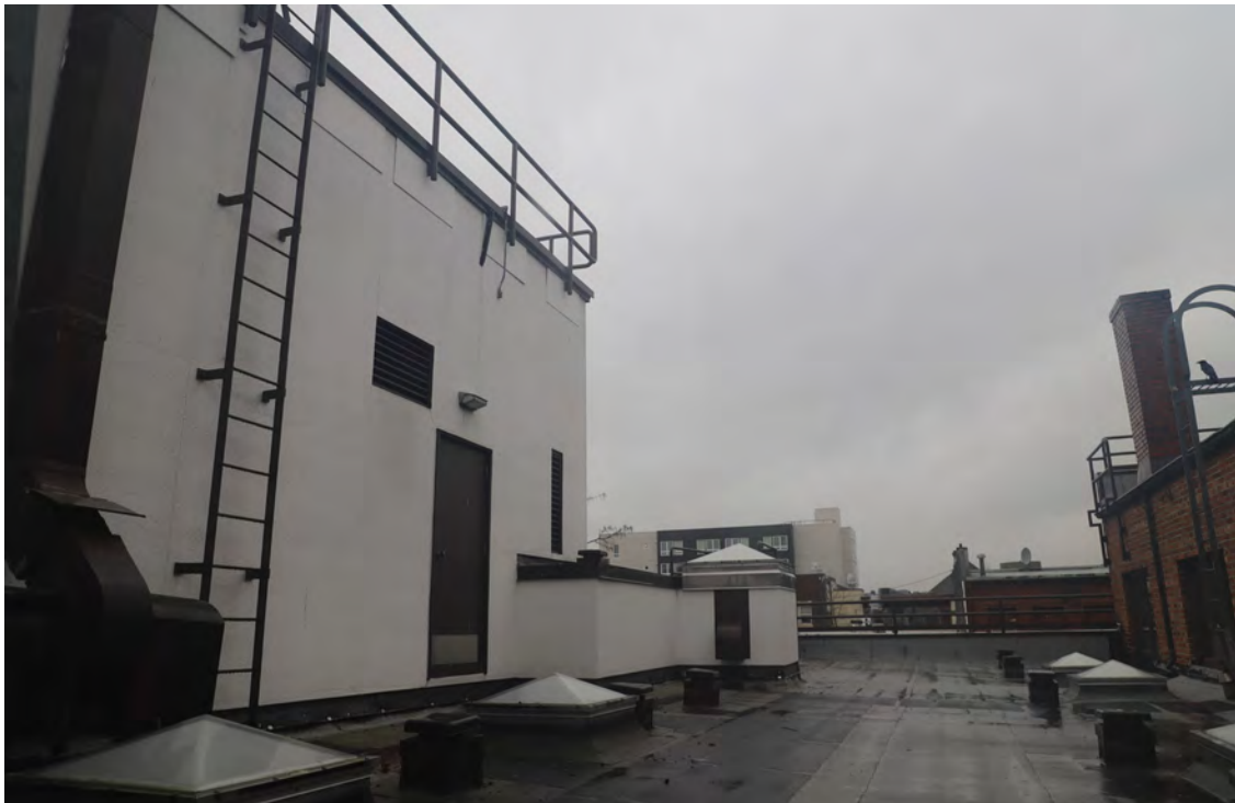
Figure 39. Roof over the southwest portion looking west. The south mechanical addition is visible at left.
