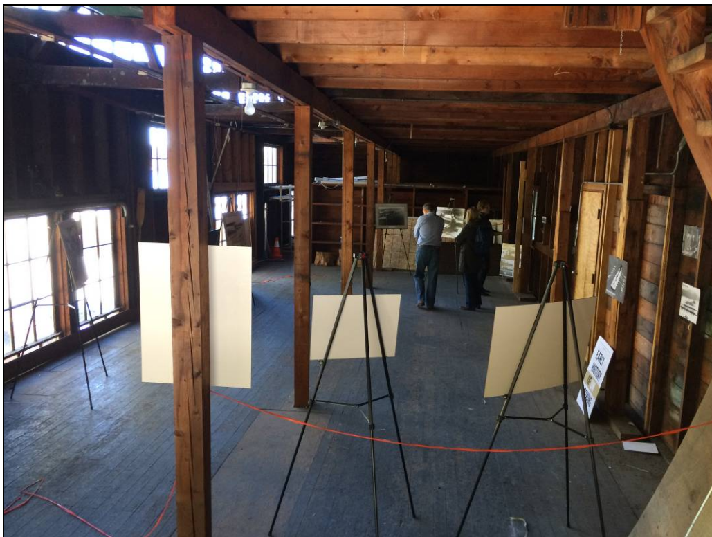
Figure 26. Interior view looking west in the mezzanine at the north end of the building.
