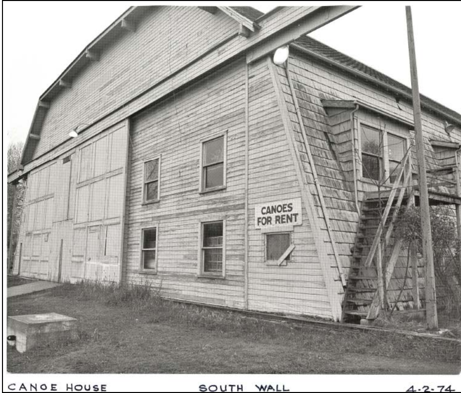
Figure 5. Exterior view showing the non-original apartment and exit stair, later removed. (UW Facilities Records)
