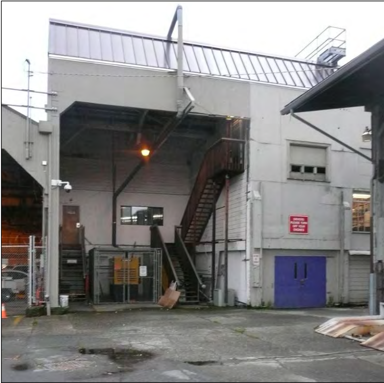
Figure 18. Above left, detail view looking west at the covered exterior space and stairs on the east side of Building B.
