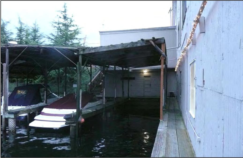
Figure 22. Above, view looking north at the south facade of Building A and a portion of Building C.
