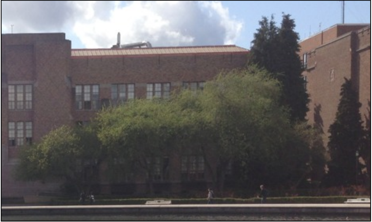
View of proposed copper gutter and mansard roof condition from Drumheller Fountain - in new copper
