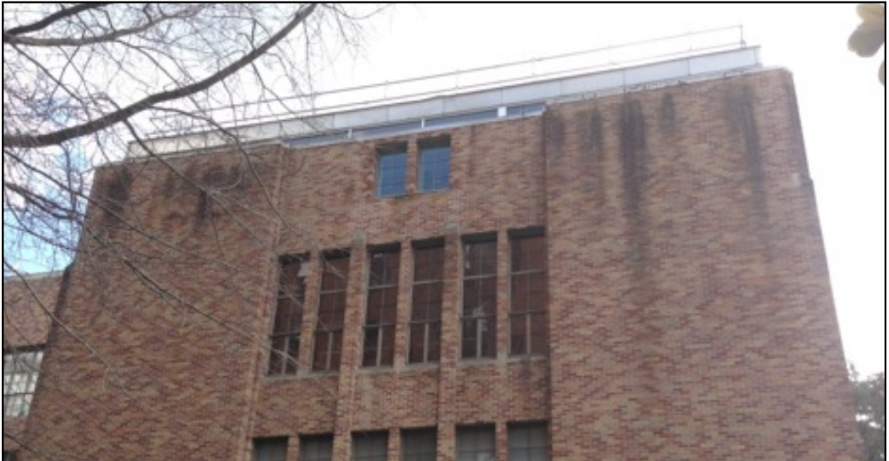
Viewing stainless steel sheet metal sheathed parapet wall at west wing from NE Thurston Lane below
