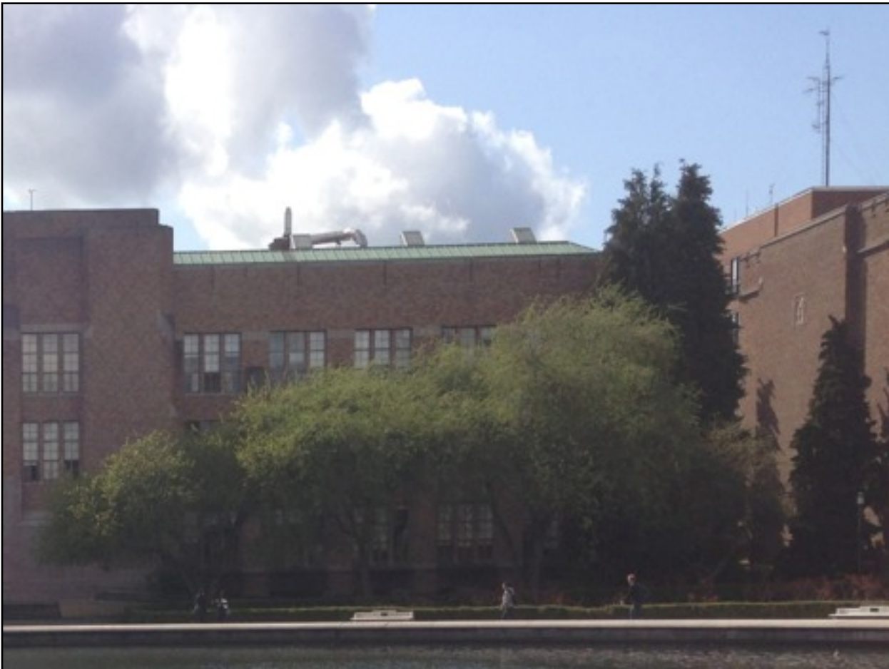
View of existing copper gutter and mansard roof condition from Drumheller Fountain
