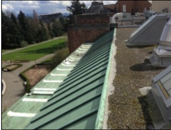
View of gutter system, mansard roof, and gravel stop from upper roof
