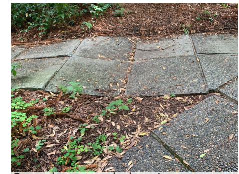
Central courtyard - heaving pavers
