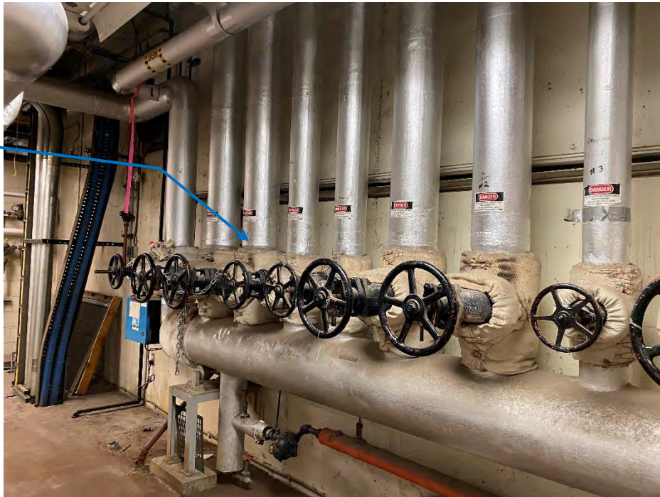
Photo 6: Ground Floor (1 st floor) Mechanical Room (north). ACM Pipe & Fitting insulation and ACM pipe valve gaskets and select blanket insulation.
