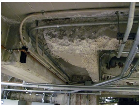
Detail under original stairs showing later pump room ceiling construction – Current Condition
