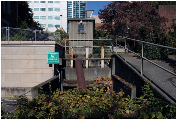
Pumphouse and Valves - Current Conditions
