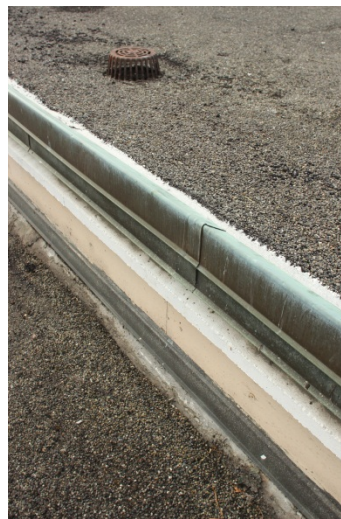
1961 Roof Edge at intersection of main roof and connector – Current Condition
