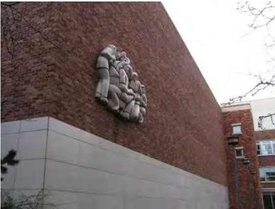
West elevation of Wing A, showing Dudley Pratt sculpture and intersection with Wing AA
