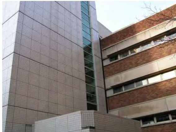
East elevation of Wing H, showing intersection of original building and new construction
