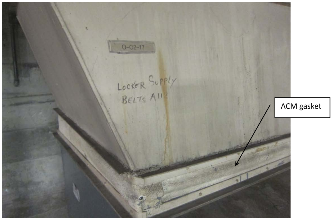
Photo 4: Asbestos-containing vibration isolation gasket associated with HVAC ductwork located in the basement mechanical room.
