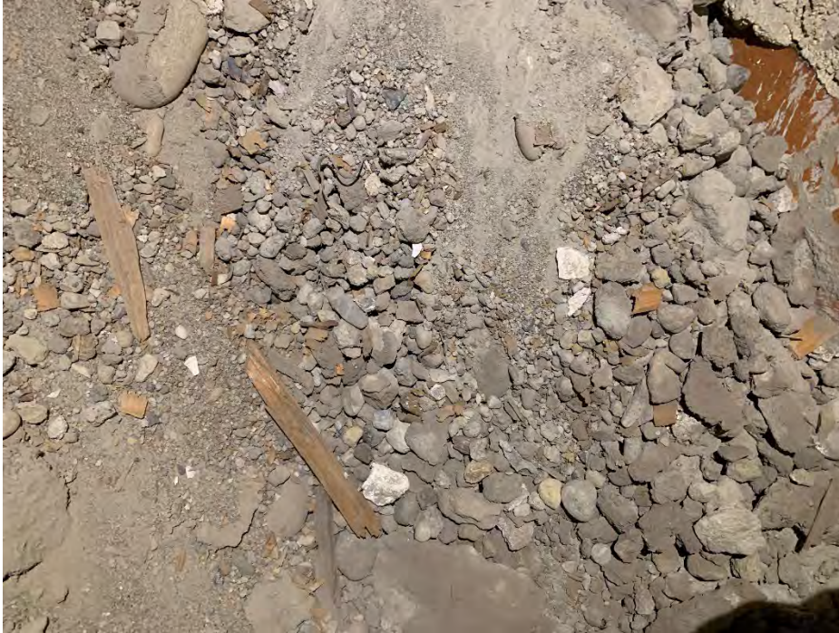
HSA 19. Gray flaky fibrous pipe insulation debris and off-white flaky fibrous residual pipe insulation debris (T)
