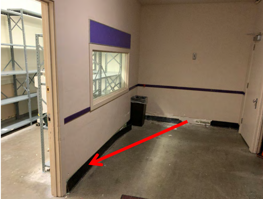
HSA 3. 6" black rubber cove base, brown brittle mastic, yellow mastic, white compacted powdery material with paint, and trace white compacted material (M)
