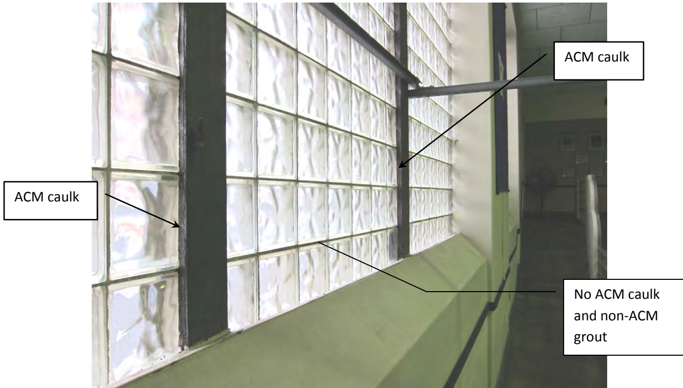
Photo 1: Asbestos-containing material (ACM) caulk (gray/tan) on glass block windows at the north end of the pool area.
