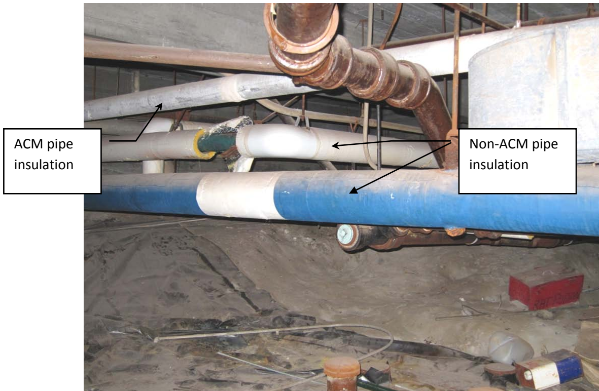
Photo 5: Basement level crawlspace with asbestos-containing pipe insulation with assumed asbestos debris present beneath the plastic sheeting vapor barrier.
