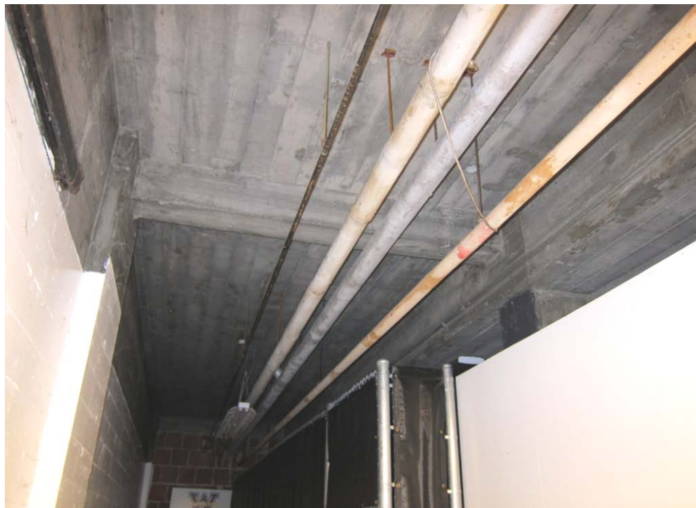
Photo 6: Asbestos-containing pipe insulation located in the ground floor east corridor.
