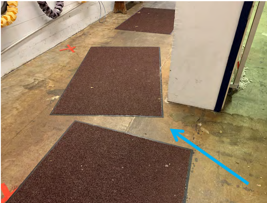
HSA 2. Off-white concrete, gray foam, beige mastic, and gray soft material (M)
