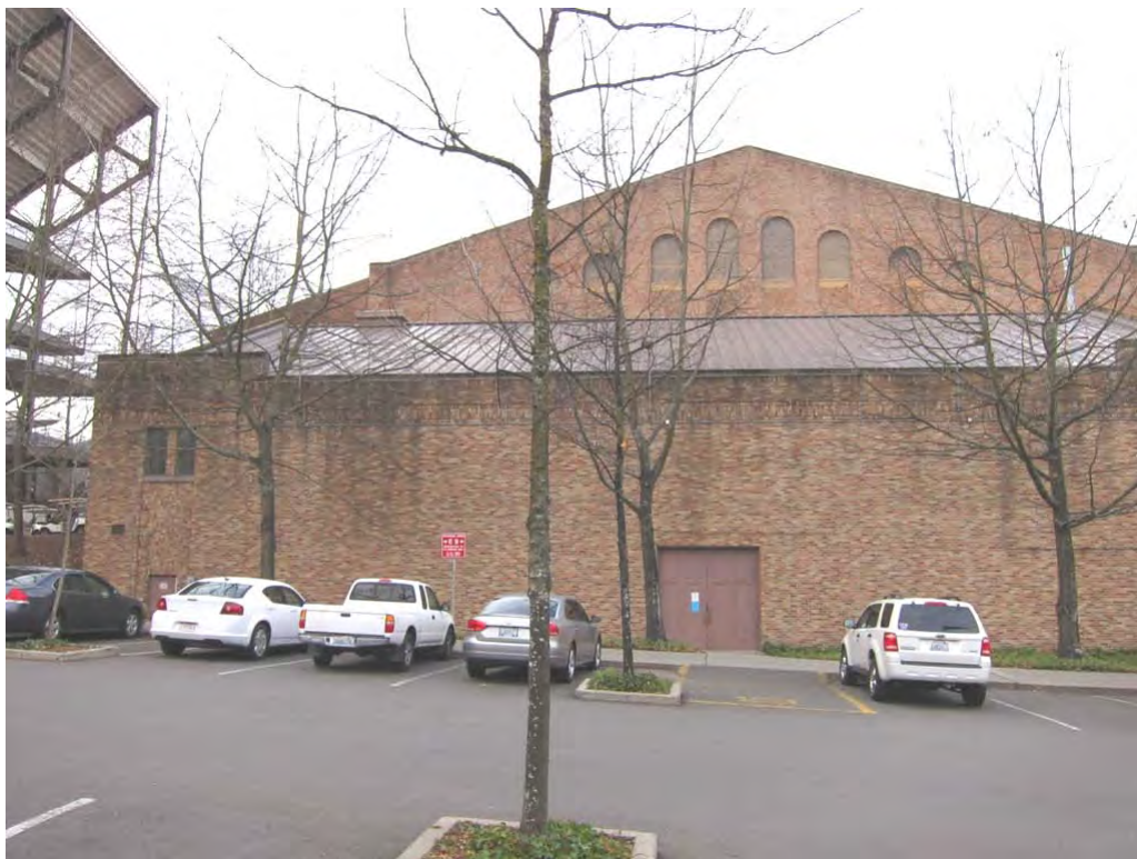
Photo 8: Assumed ACM vapor barrier or coating behind masonry brick façade of the Pavilion Pool building.
