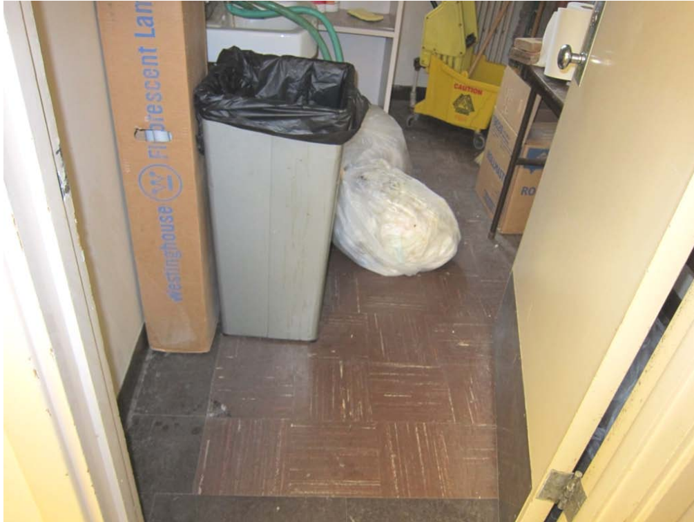
Photo 3: ACM 9" vinyl floor tile and mastic (dark brown) in the pool building.
