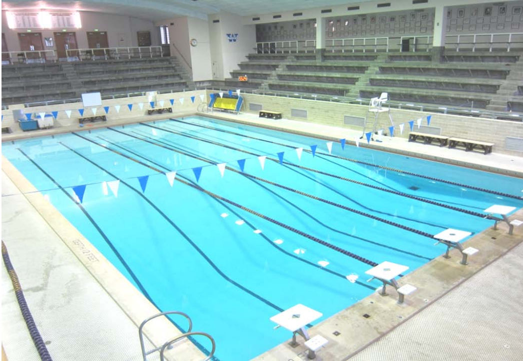
Photo 7: Assumed ACM vapor barrier or coating underneath the pool walls and floor.
