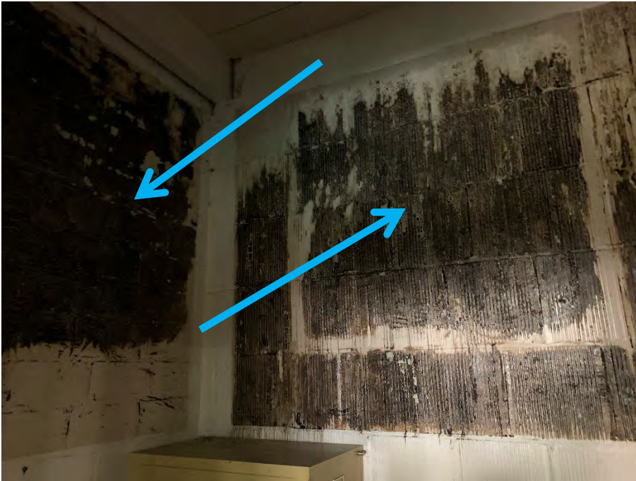
HSA 10. Black residual mastic with paint (M)
