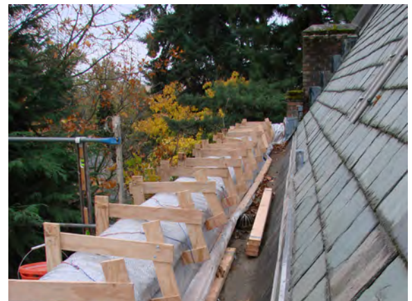
Water Penetration Investigation
