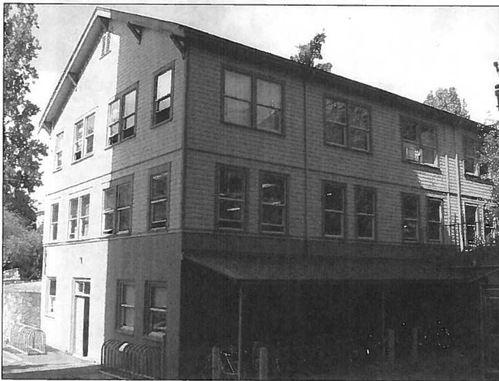
Looking northwest, showing the south facade and southern portion of the east facade.
