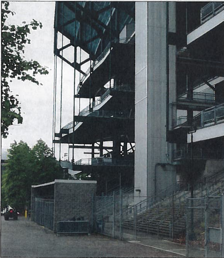
Husky Stadium North Stands, partial oblique north elevation. Note central elevator tower and cable-suspended access ramps.
