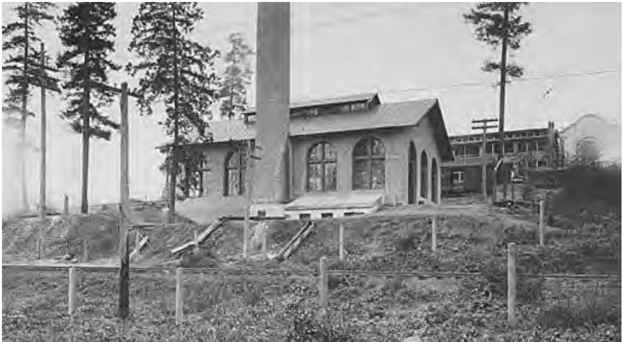
Figure 23. Ca. 1908 view during construction of the Foundry taken from east of Power House #1 (in the foreground) and looking west with the northeast end of the Foundry Building visible in the background and a portion of Machinery Hall visible behind the Foundry. Photographed by Frank H. Nowell. University of Washington Libraries, Special Collections, Negative Number Nowell x769.
