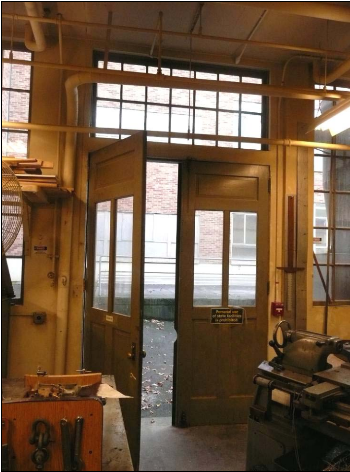
Left: View of exit doors and wood transom windows on the west side of the first floor wood shop (Room 128). The doors and fenestration appear to date from the original 1920 era of construction.
