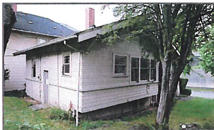
Field site no. 4 rear (east) and side (north) facade view. Source: Artifacts Consulting, Inc. 2008.
