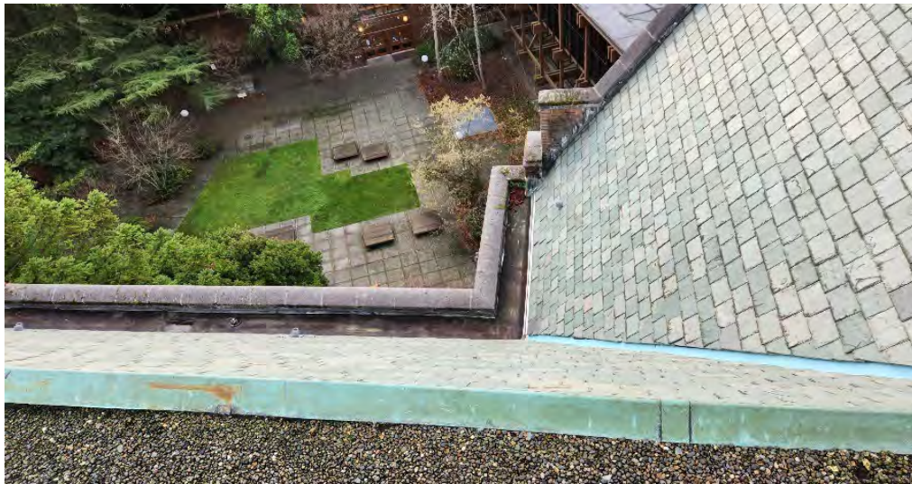
Photo 12: ACM built up roofing around the roof gutter area and parapet wall.
