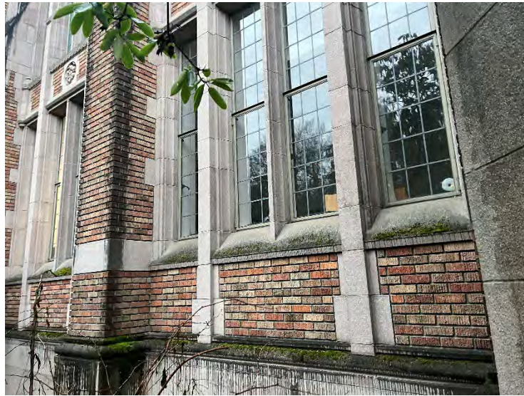
Photo 9: PCB containing grey rough opening caulk at windows. Barium and lead containing brick and mortar.
