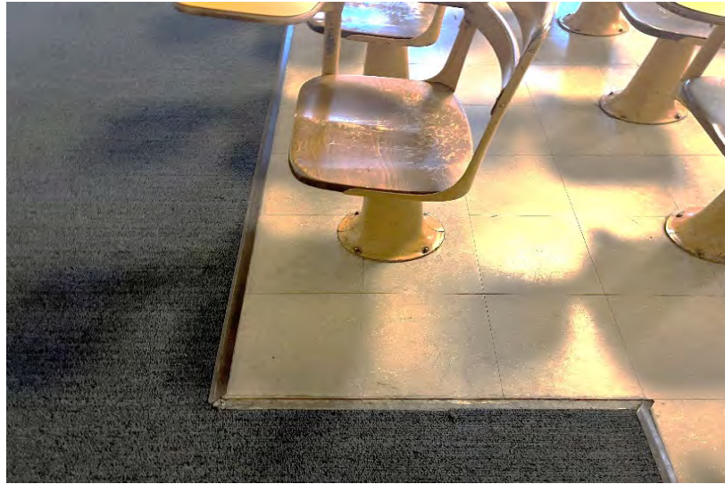
Photo 1: 12"x12" beige floor tile with ACM black mastic in room 223. Beige 12" tile and black ACM mastic throughout the ground, first and second floor.
