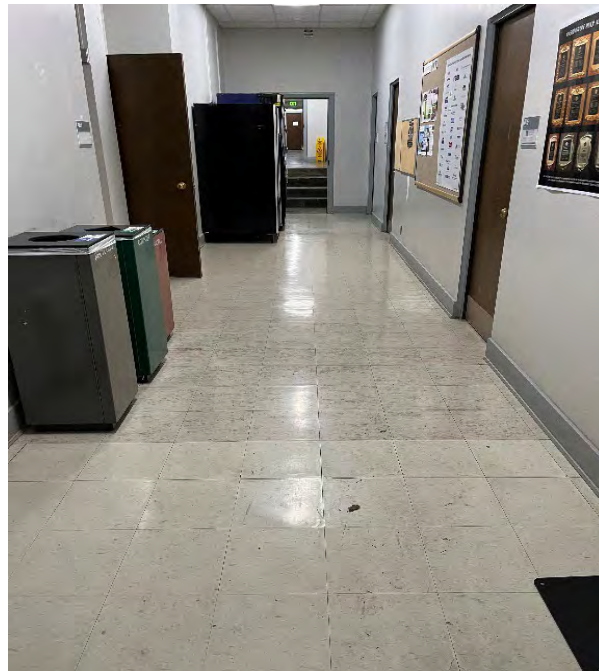
Photo 2: 12"x12" white/off-white and beige floor tile with ACM black mastic in ground floor hallway. Beige and white/off-white 12" tile and black ACM mastic throughout the ground, first and second floor. Assumed less than 1% of asbestos (wallboard/drywall and joint compound composite)
