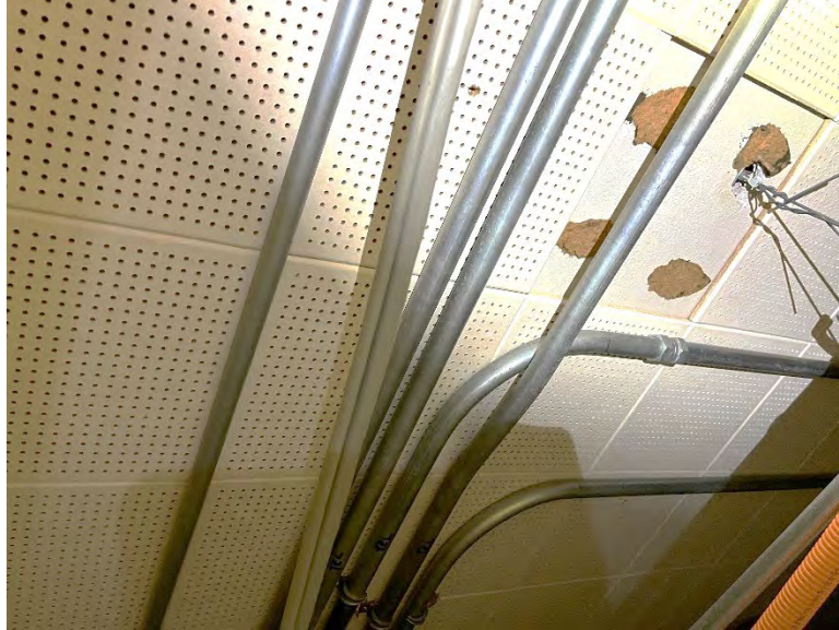
Photo 5: Non ACM 12"x12" glued on ACT above dropped ceiling in room 123. ACM glue dots.
