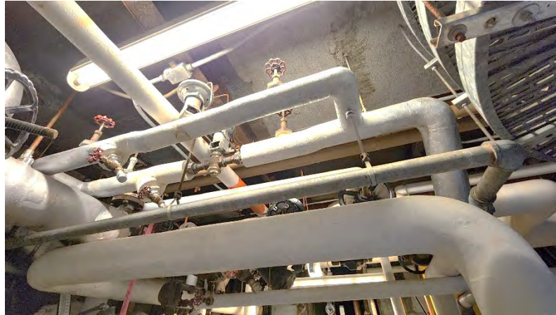
Photo 7: ACM hard fittings and straight runs present in basement mechanical room accessed from south exterior side of building.
