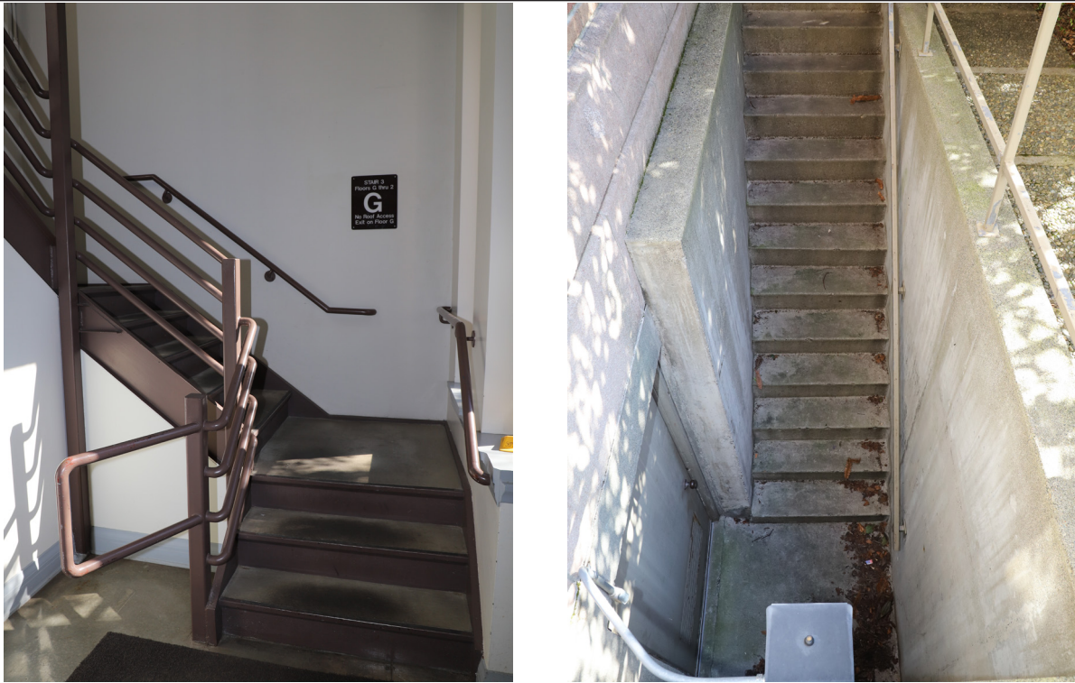
Figure 53. Southeast stairway at the first floor (left) and the exterior basement stairway (right).
