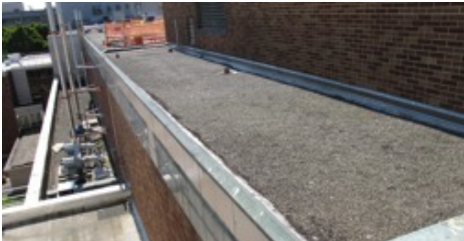
Roof C1 and C2 with high parapet conditions on the left and roof D4 with a gravel stop.
