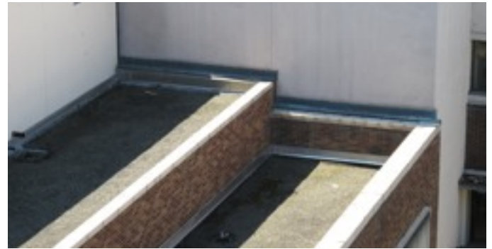
Roof F7 on the left with a low parapet is not visible from below, and F8 has a high parapet.
