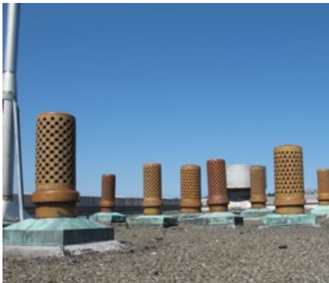
Existing vents on D5, notice the new vent at left.
