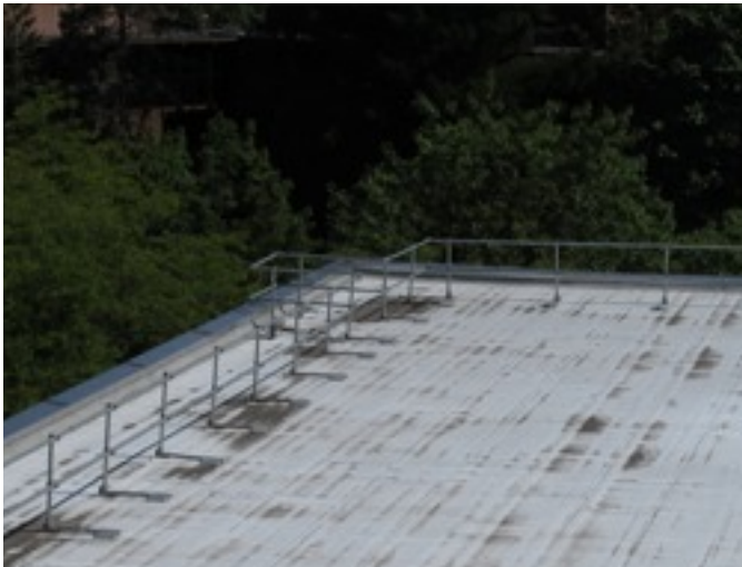
Safety railing on A wing.
